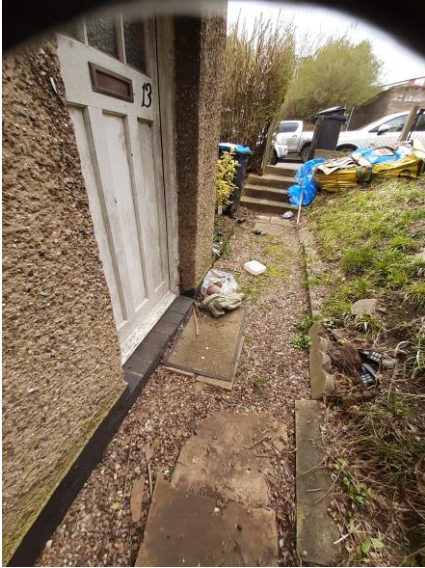
Condition of front door
